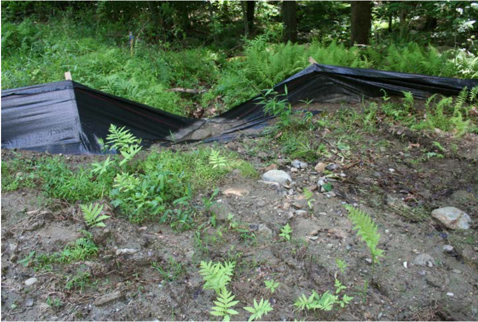
Filter-fabric silt fence overtopped by storm flow draining into Wetland A-34, photographed 9 July 2014. Photograph looking downhill from the pipeline right-of-way just east of Stoney Street.
